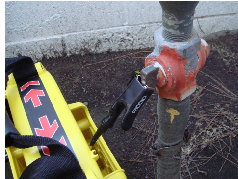
Figure 7 – Cable Lead clipped to target conductor
